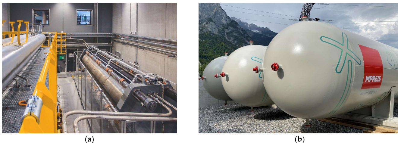
Figure 7. (a) PAE supplied by Sunfire GmbH at the right and the gas separators at the left; (b) three hydrogen storage vessels supplied by APL GmbH (Tyrolean company), with permission from MPREIS.
